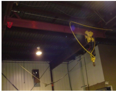
6 Ton Overhead Crane
